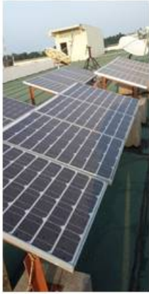
Solar Panels (1.5 kW)
