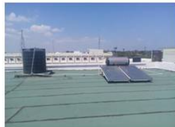
SOLAR WATER HEATER
